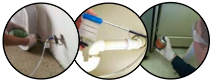
Dust outlets, plumbing, voids
